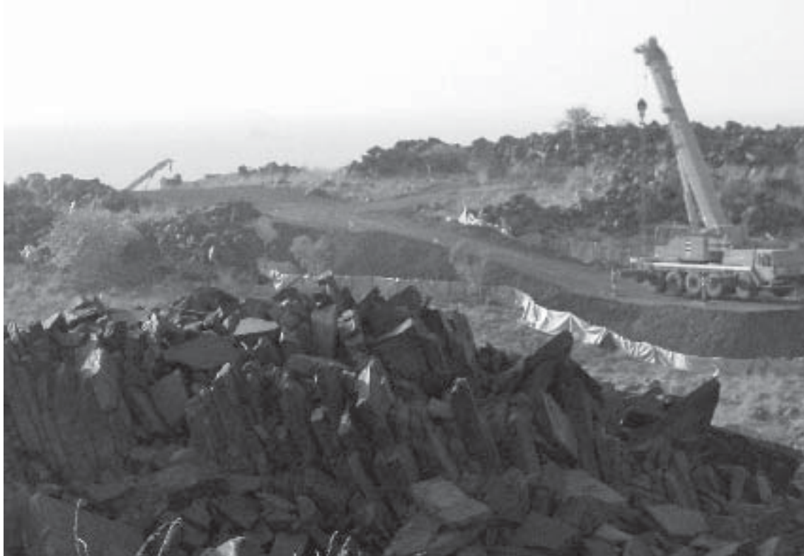
Figure 6. Mobile crane setting up to remove petroglyph boulders, February 2007, Site A at Holden Point.
