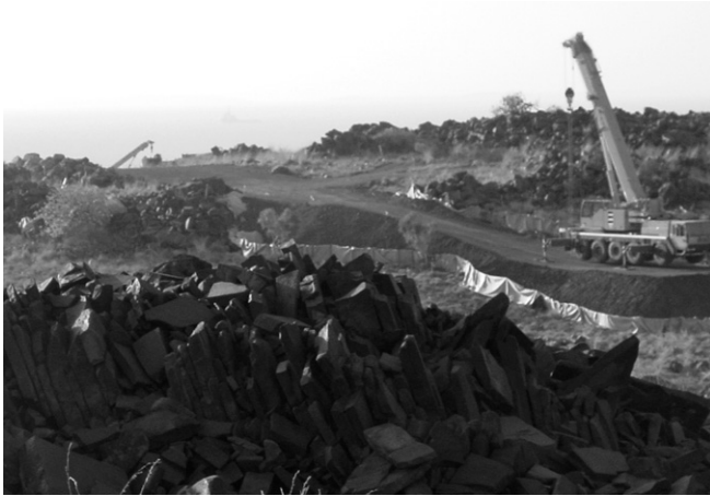
Pluto plant site, Dampier Archipelago, January 2008. Two massive cranes on temporary roads remove rock art. The operation cost in total about $5 million, so you can imagine its scale.
