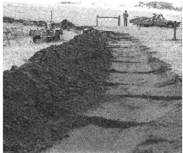
Figure 5. South-eastern section of the drainage channel constructed. The stock fence to enclose the reserve is also under construction.
